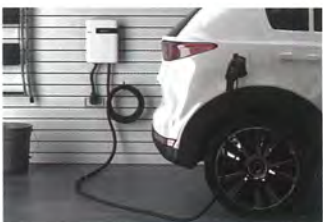
Electric Car / Fast Charging
